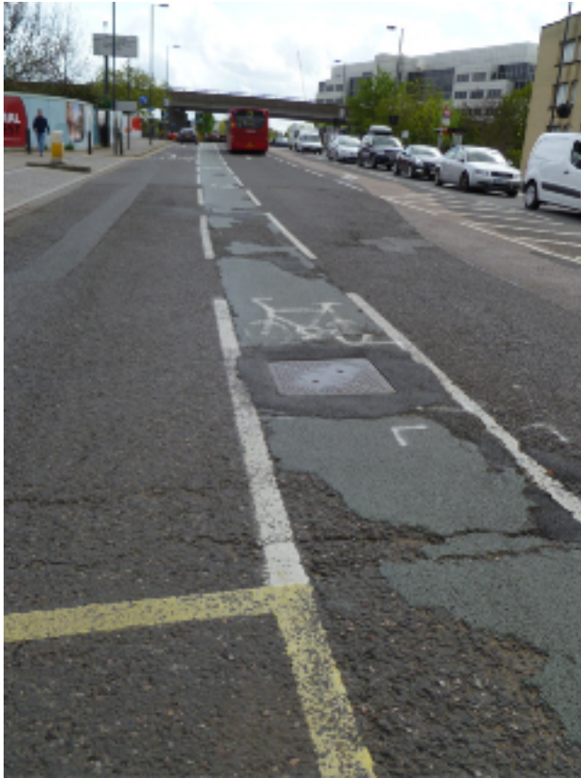
Poor road quality on Wood Lane
